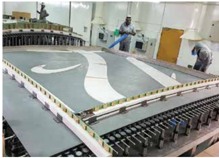
1 CNC-cut foam placeholders were laid onto the curved Adapa mold to produce the panel's A surface that visitors see.
