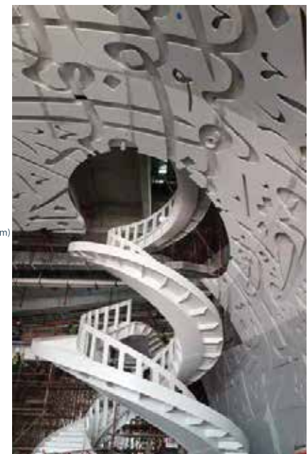
7 Panel joints (clearly visible here) were filled with FR epoxy adhesive, overlaminated and ground smooth before the final coat of paint was applied and LED lights were installed.
